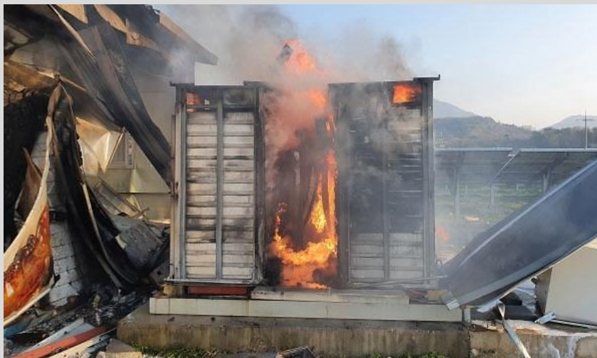
LG Energy Solutions ESS
