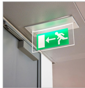
LED emergency evacuation signs
